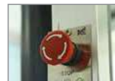
Emergency Stop Button
